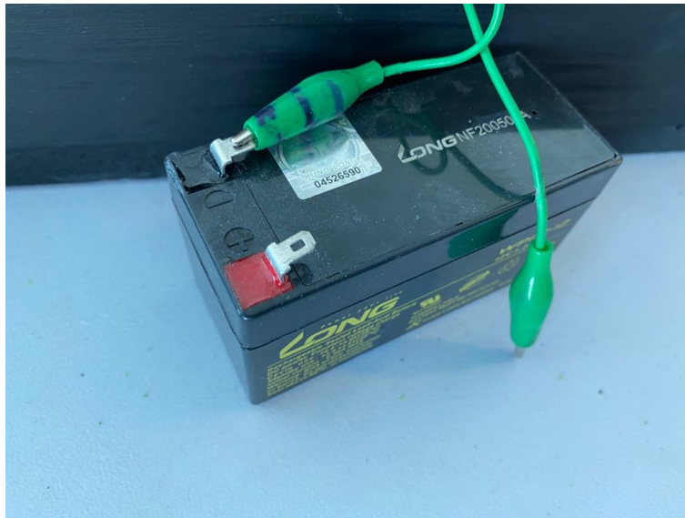
Figure 45 12V Battery Connected to the Charge Controller
